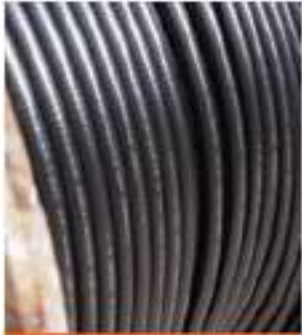
TWM feeder cables
