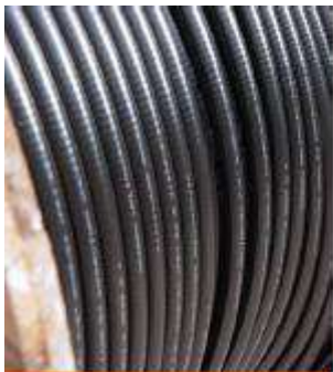
TWM feeder cables
